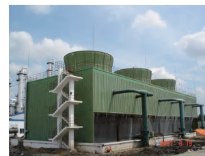
Concrete Cooling Tower
